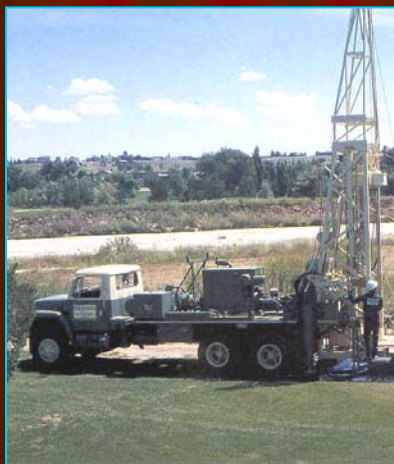
Failing Truck Mounted Rig
