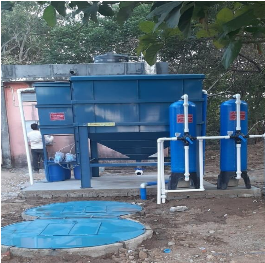
Fig 3: Photograph of 40 KLD ETP installed at Sapphire Hostel
