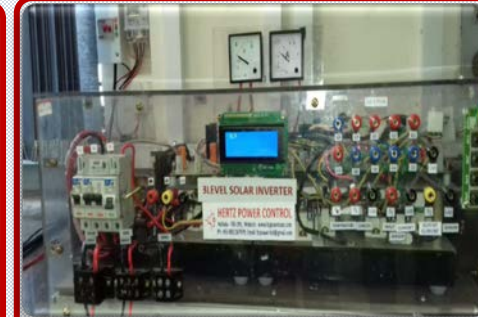
Grid Connected Solar Converter (Multilevel) System Make: Hertz Power Control
